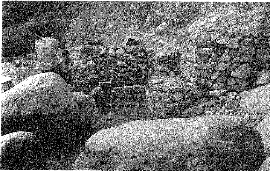
Photograph 1C Side Intake Built Between Large Boulders
