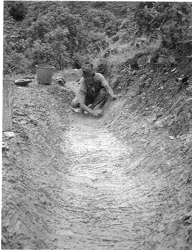
Photograph 7D Village Worker Plastering an Earthen Canal with a Mixture of Soil-Cement
